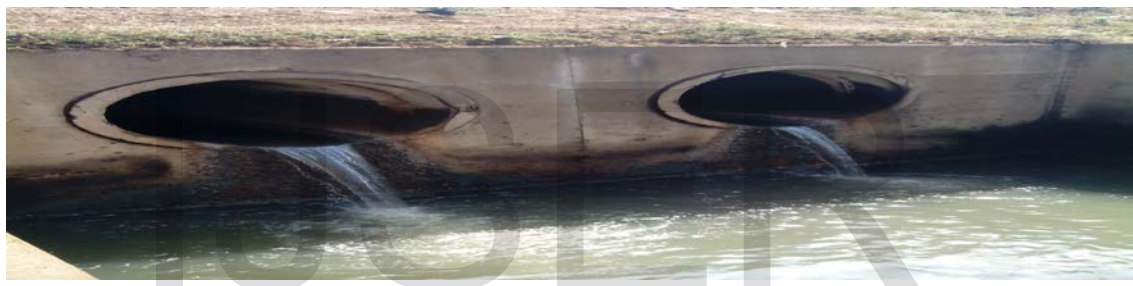
Figure 2.5. Effluent outfall from the Refinery.
